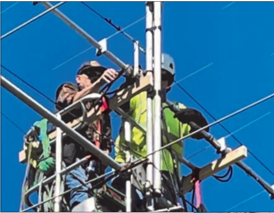
Those are 2x4's carefully strapped to the "bucket" to hold/carry/lift each antenna
